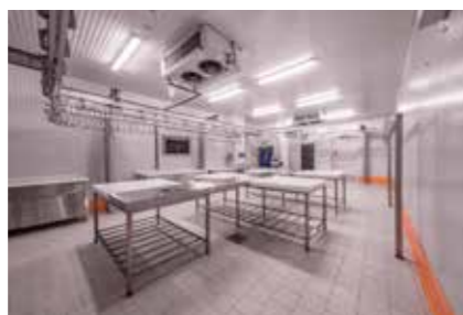
Industrial storage (refrigerated warehouses and producing areas)
